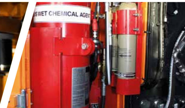
Automatic fire suppression system
