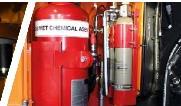
Automatic fire suppression system
